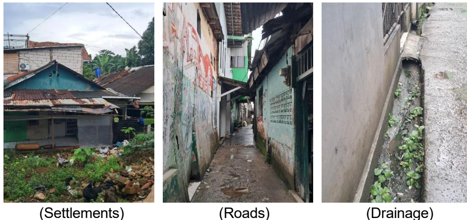
Figure 1 Current condition of infrastructure in RT 07 Babakan Raya
