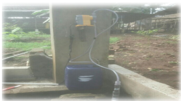
Figure 1. Dosing equipment using hydrogen peroxide disinfectant
